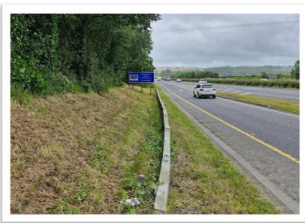
OBB barrier at former high lighting mast and cutting slope to rear on M1 slip on approach to the nosing with the mainline.
